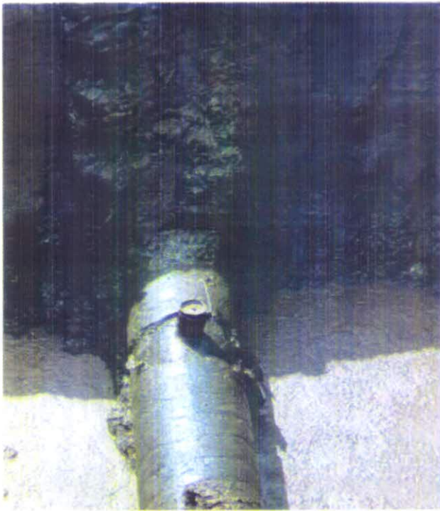
Figure 1. EXPOSED INCIDENT POINT
